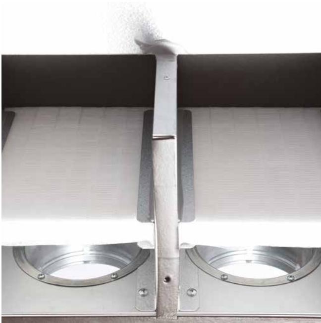
ISO ePM1 filters positioned inside heat recuperator.
